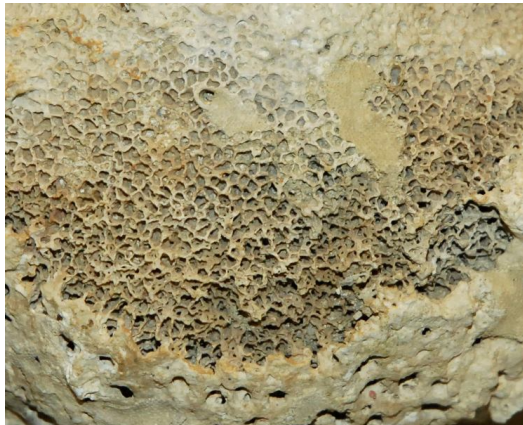
7. The eroded surface of a stone ball (Photo: M. Ćurković)
