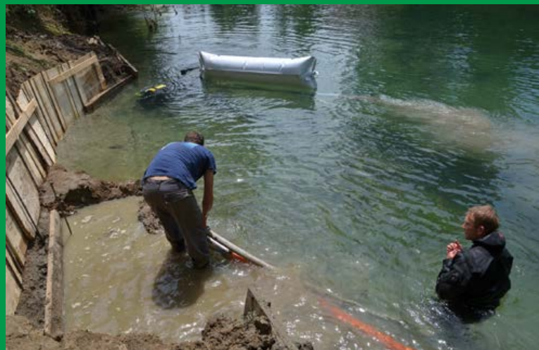
3. Excavating simultaneously above and under water / Sočasna izkopavanj nad in podvodo (Photo: D. Pavlovič)
